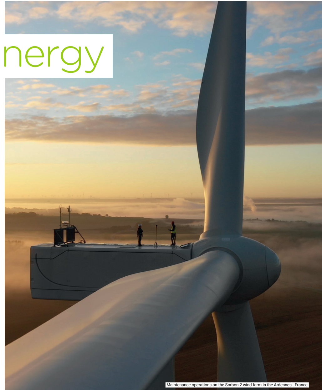
Maintenance operations on the Sorbon 2 wind farm in the Ardennes - France.
